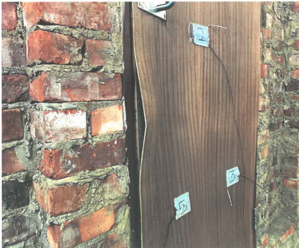
Photo 5: Door face loosening
