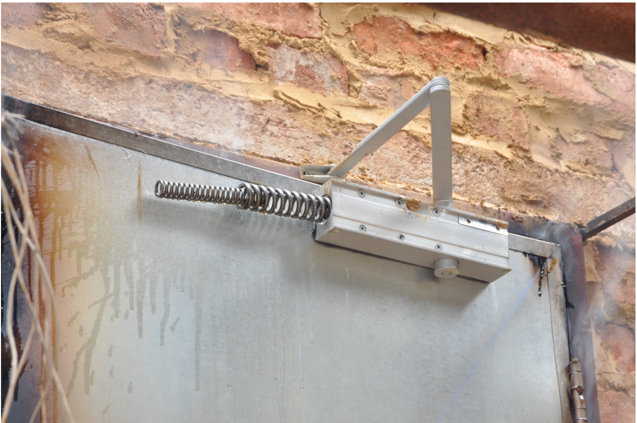
Figure 4.2.8: Door closer rupture
