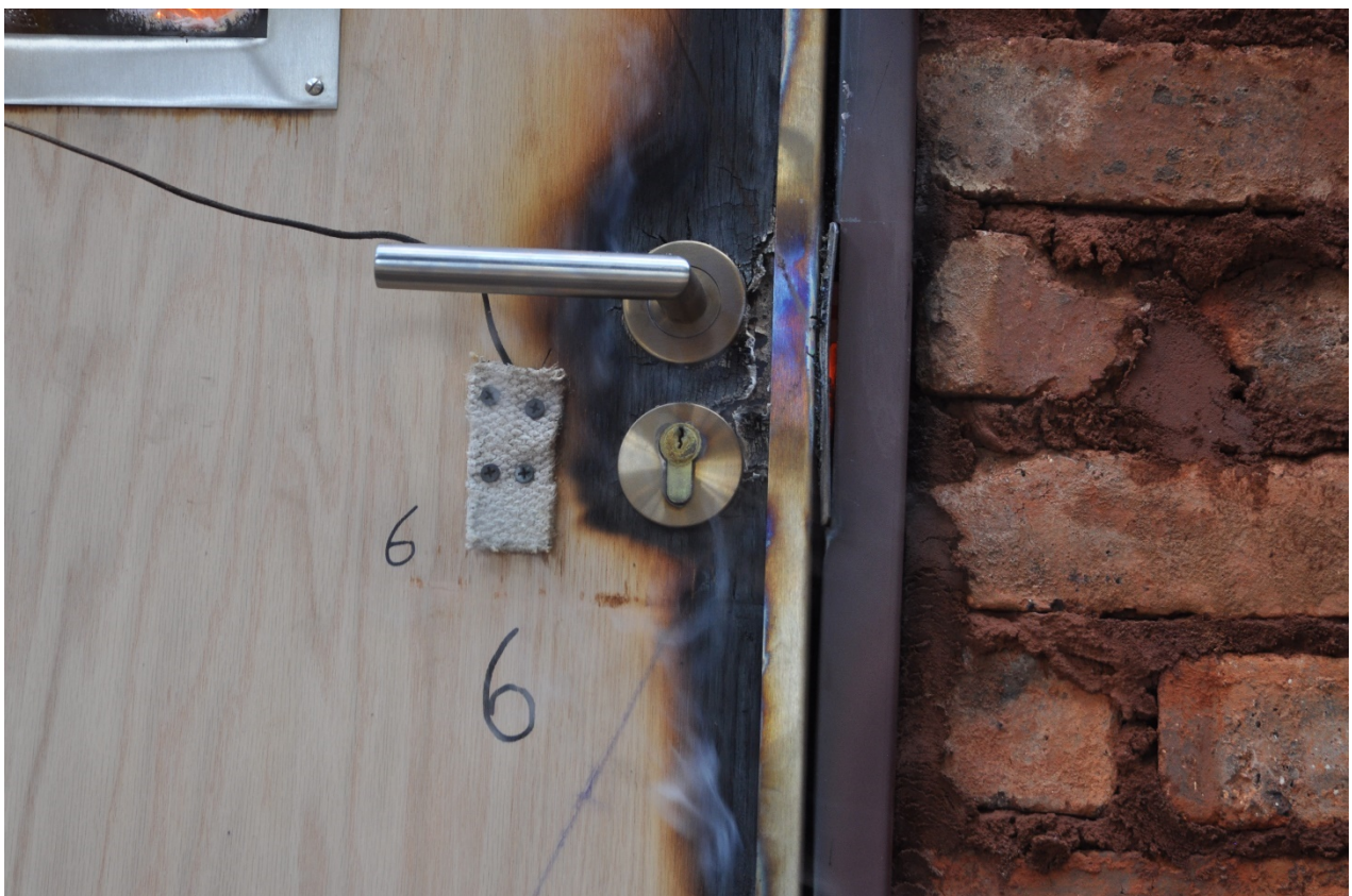
Figure 4.2.16: Discoloration on steel near lockset
