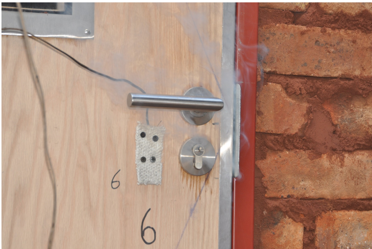
Figure 4.2.7: Discoloration at lockset
