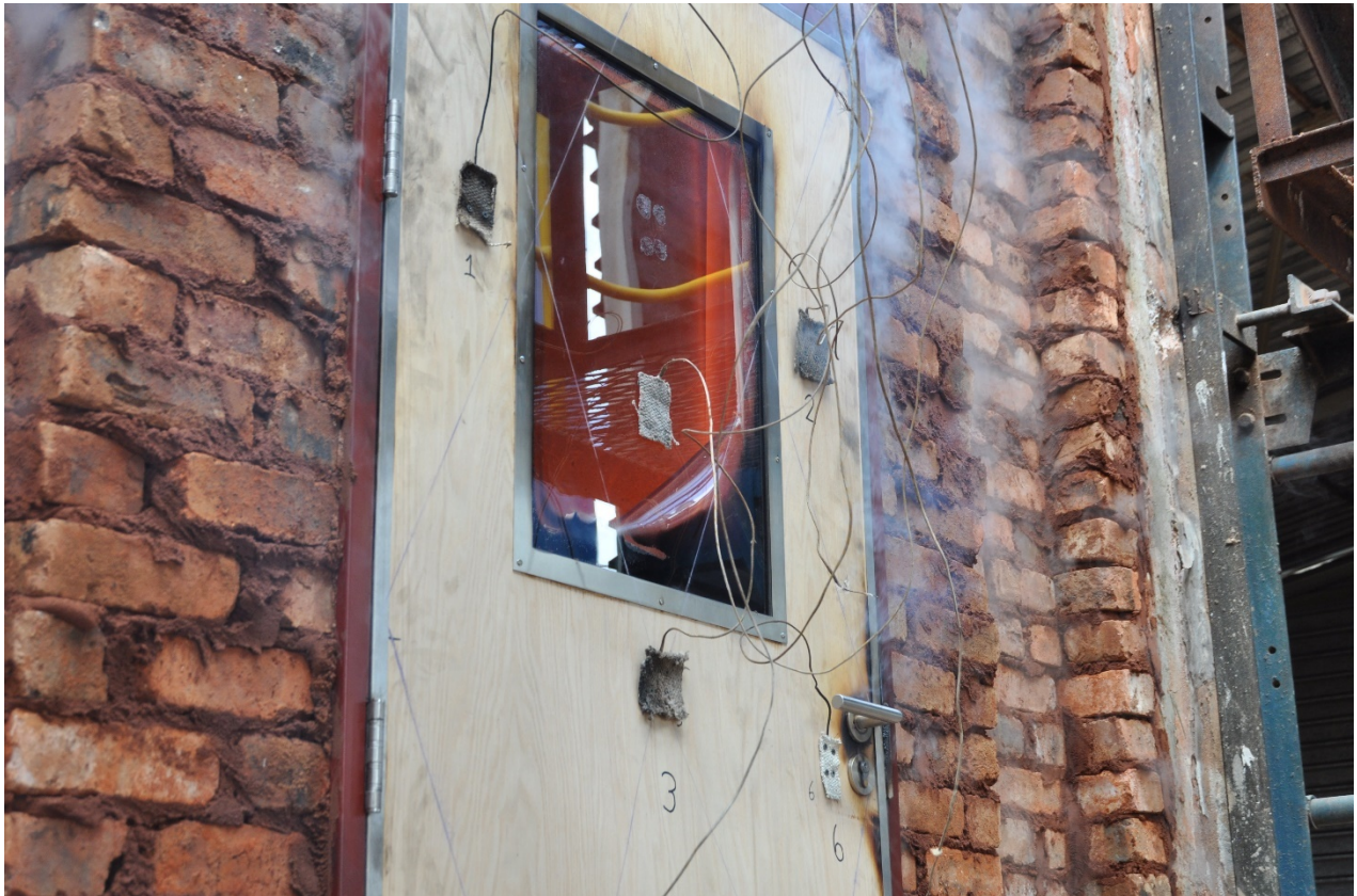
Figure 4.2.13: Glass on exposed side melted
