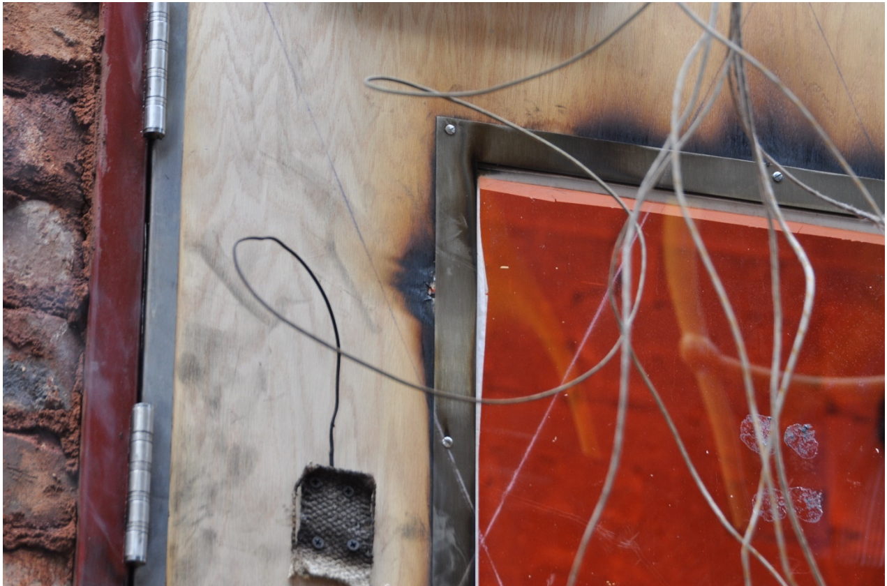
Figure 4.2.15: Glowing on timber, left of glazing (view panel)
