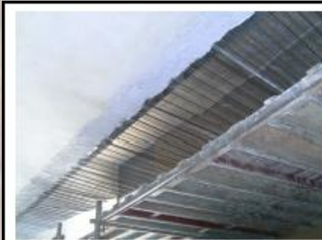
P&H Rocklite 'GC' 2 Hour Fireproof Ceiling, Bottom View of Rocklite 'G' Plaster and Riblath Sheet.
